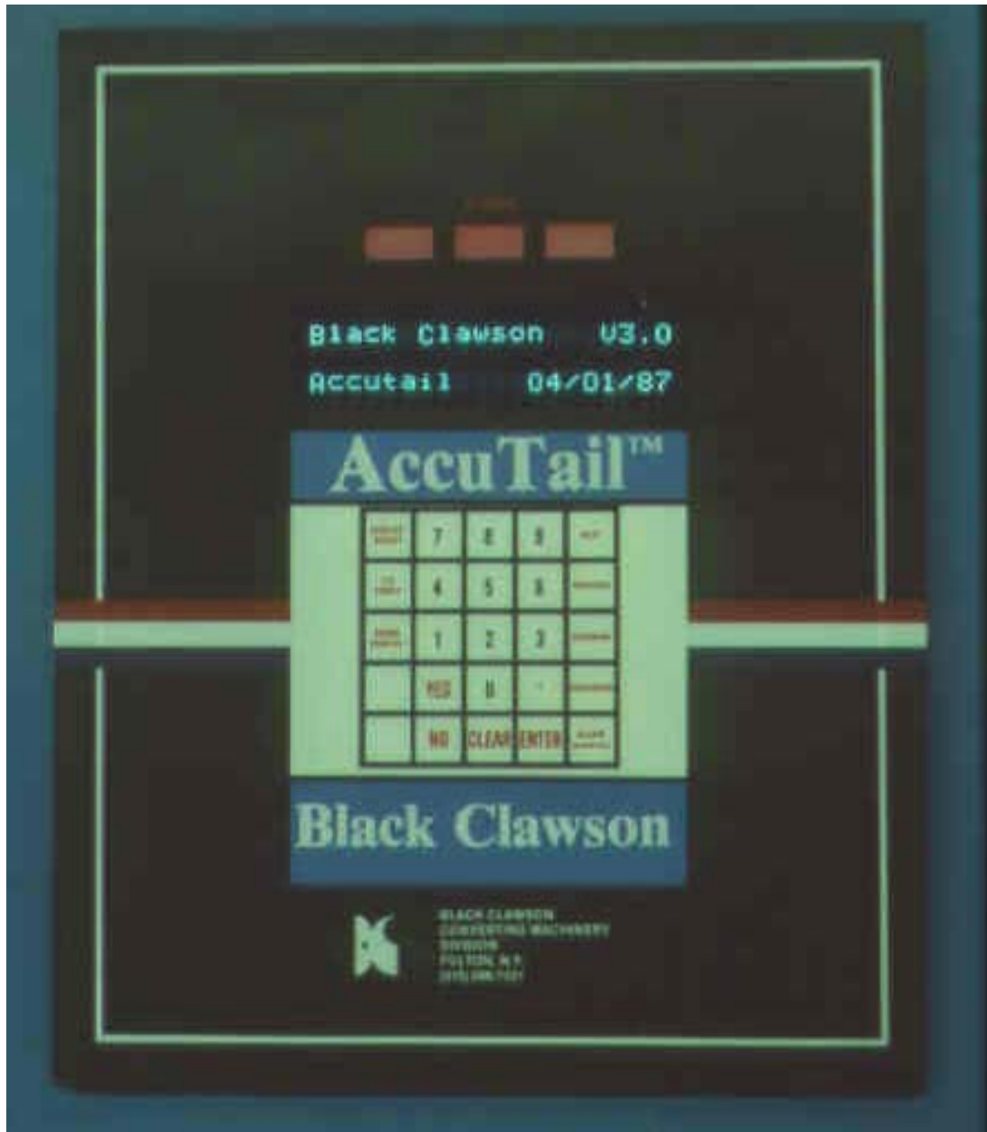
Typical Microprocessor Operator Interface Panel
